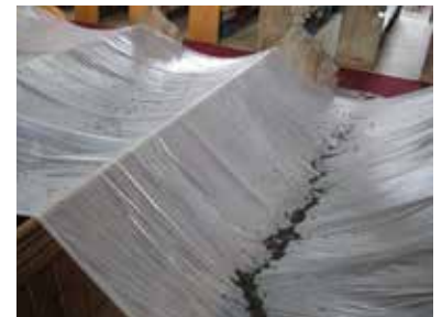
Bat droppings accumulated over a short period of time on protective sheeting.
