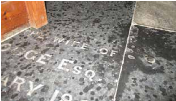
Bat urine stains on a church stone floor.
