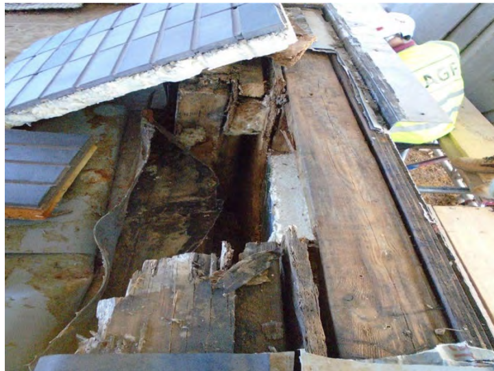
Figure 2.8: Building Pathology from Use of Impermeable Membranes and Insulation
