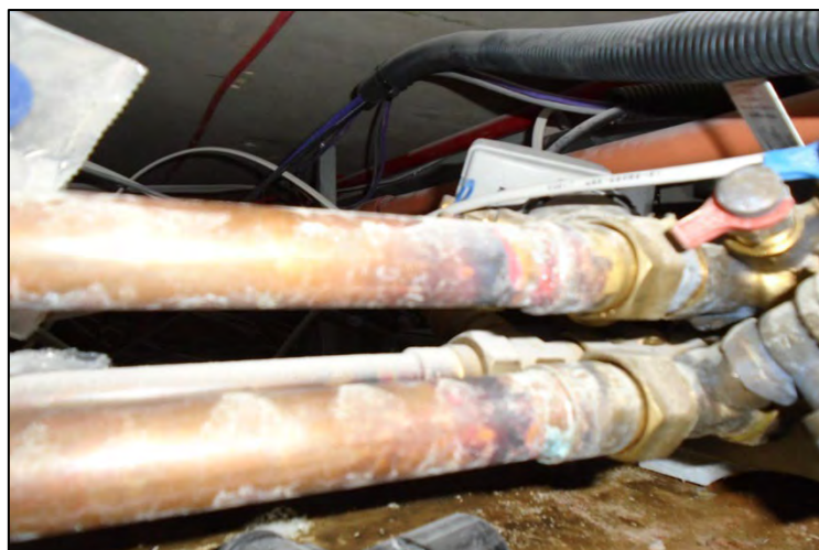
Figure 2.7: Emergent pathologies in Heating and Ventilation
