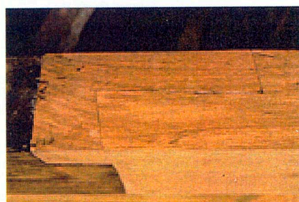
A short scarf joint on an oak panel moulding at Kingston Lacey, (McCurdy & Co, for the National Trust)
