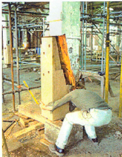
Scarf repair at the mast house and mould loft, Chatham Historic Dock Yard (McCurdy & Co Ltd)
