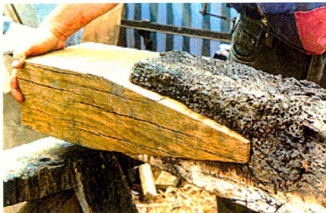
Weald & Downland Museum: New oak repair to a death watch beetle decayed post, ensuring the retention of the maximum amount of the original material. (Hutton+Rostron)
